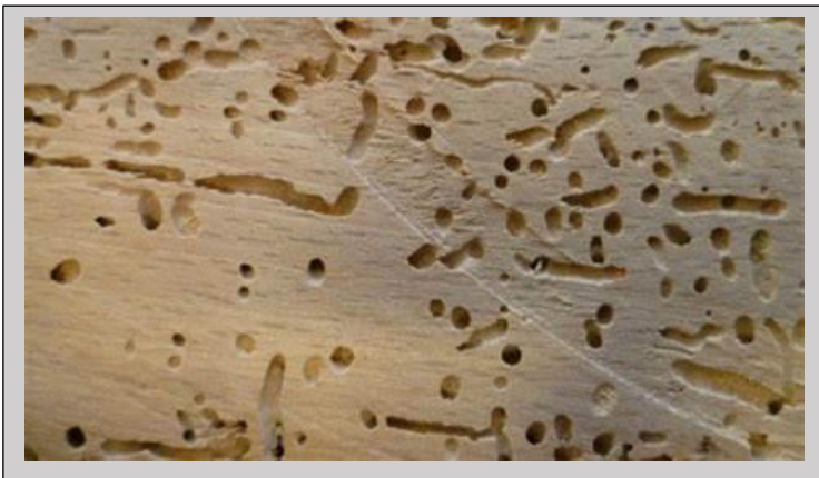
Flight holes indicate that this wood has been heavily infested with the common house borer.
